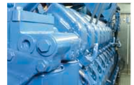
Powerful diesel generators supply constant, reliable power.
