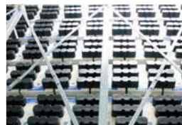
Lead gel batteries guarantee continuous power without interruption.
